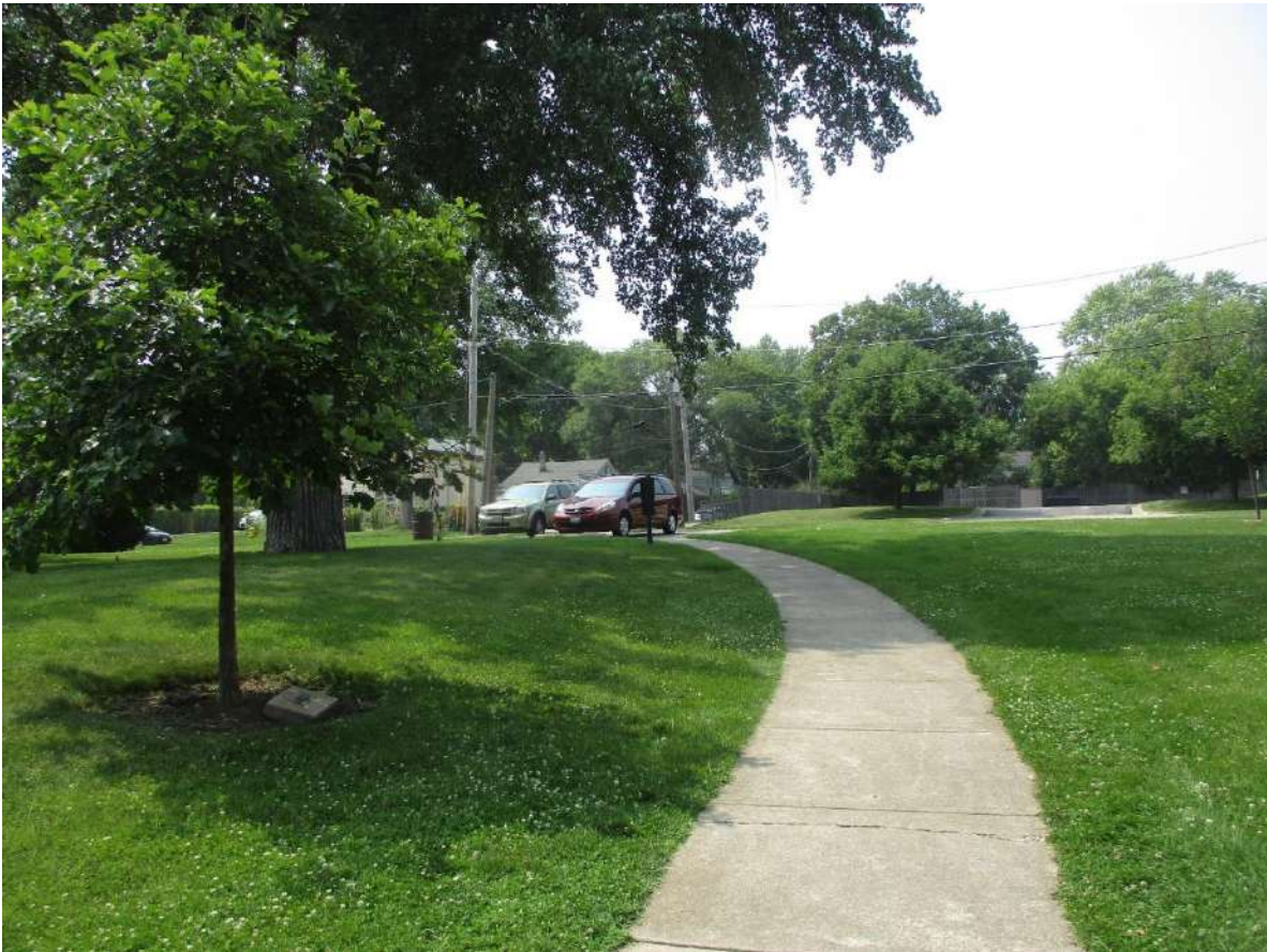
Remove and replace one concrete square that is cracked between parking lot and playground = 5' x 5'
