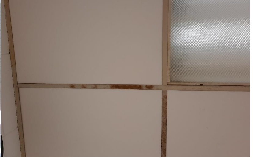
SAMPLE OF RUST ON CEILING GRID
