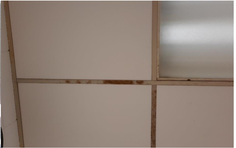
SAMPLE OF RUST ON CEILING GRID
