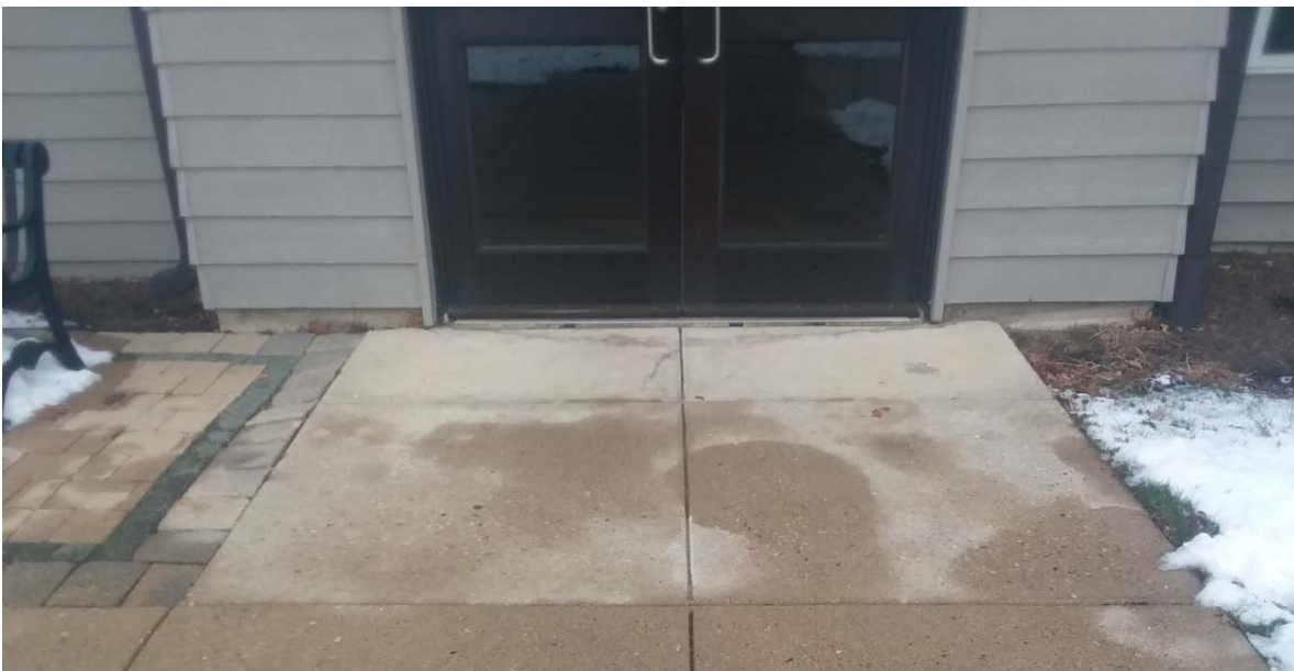
Existing concrete at Jack Benny Entrance to be addressed with Alternates 1 and 2 -
