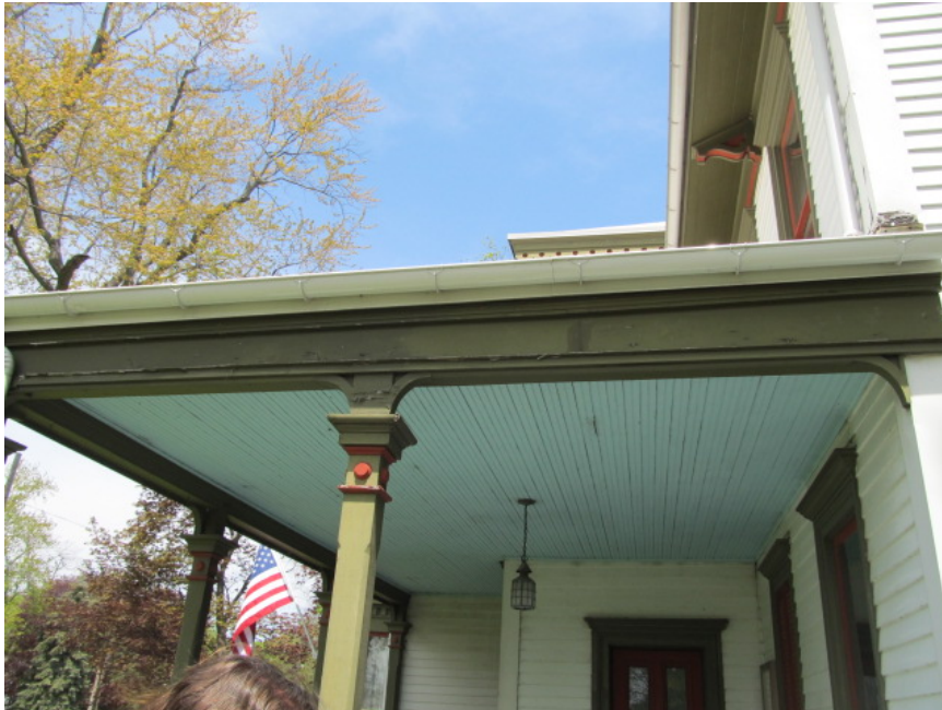
Replace top drip cap 14’ along the south side of the front porch
