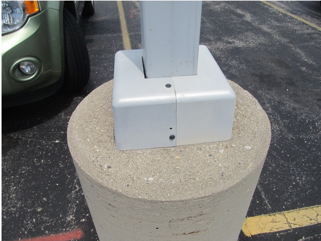
Paint area under Caps at Base of Lights
